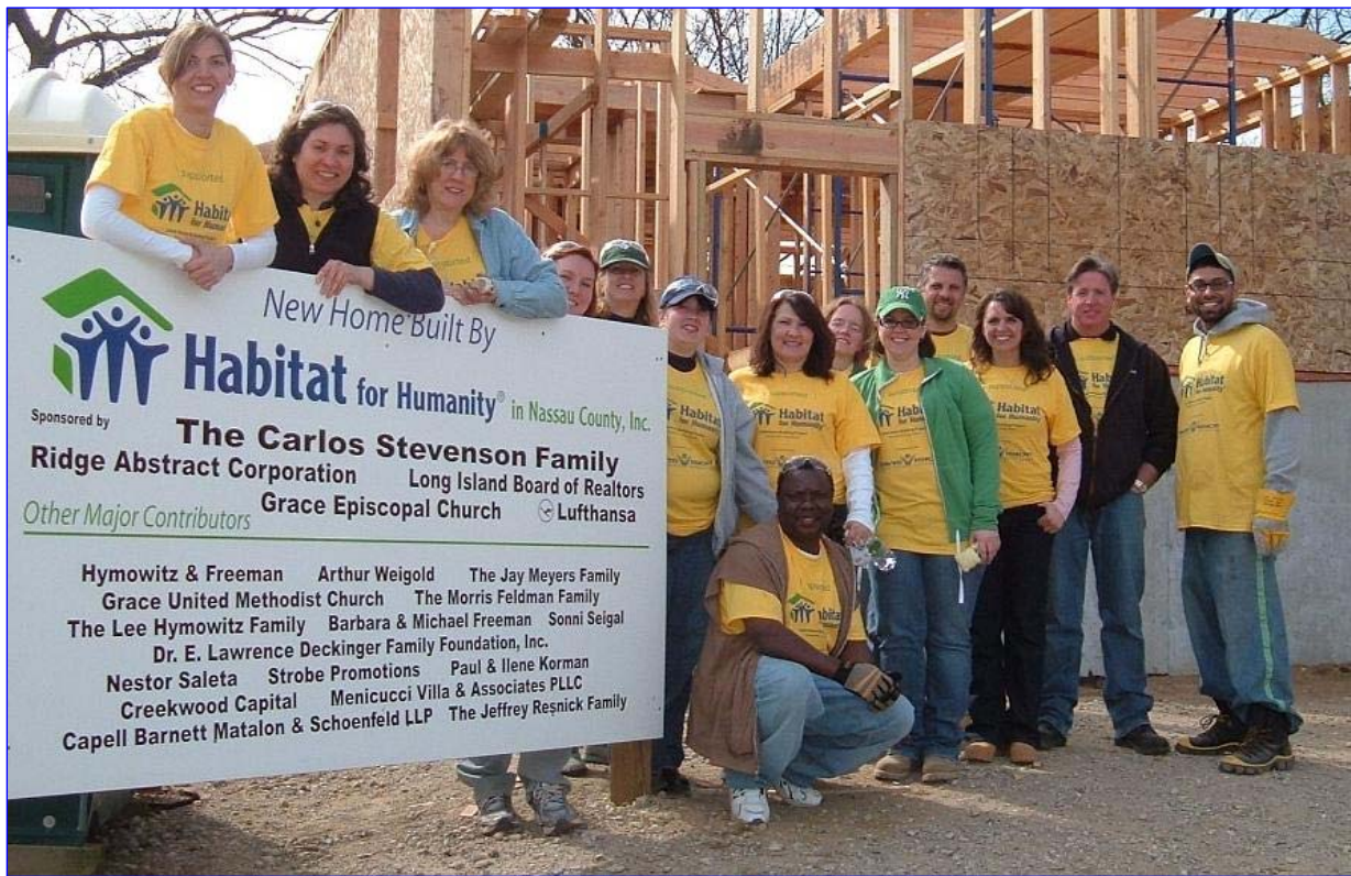
Davis Vision employees spent weekends helping to build a Habitat for Humanity house on Long Island, NY.
